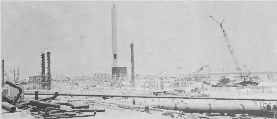
The first towers and the furnace for the Vacuum Pipestill are set in place. E promer towernan y forno pa a Vacuum Pipestill ta ser poní na nan lugar.
